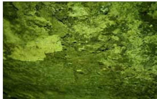
Photo.1 Exfoliation of concrete on inner lining
